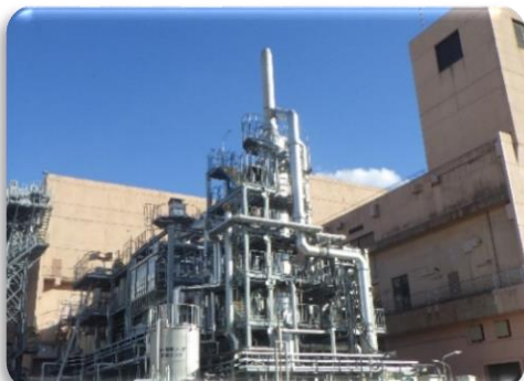
⑨ 汚泥焼却設備 (70t)
