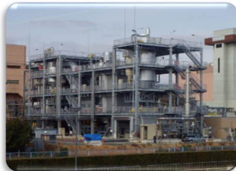
⑩ 汚泥焼却設備 (110t)
